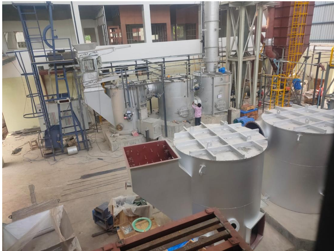
A site visit to study Air Pollution control Devices Design and Manufacturing
