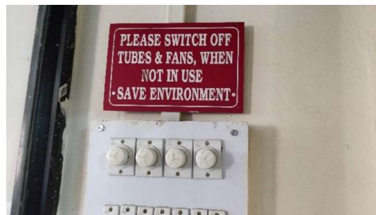
Typical display board near each switch board
