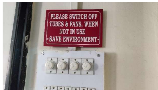
Typical display board near each switch board
